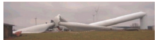
Collapsed wind turbine tower due to fatigue cracks and wind loading combination.
